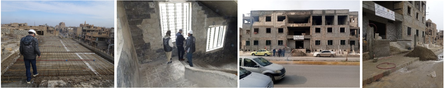
Above: Before and during rehabilitation of the Cadastral Affairs building in Deir ez-Zour
