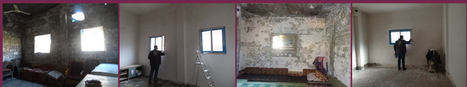
Above: Before and after rehabilitation in apartments in Al Omal, Deir ez-Zour
