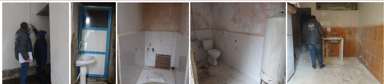
Above: Checking the new electrical system; new sink and door for WASH facilities, newly installed Eastern and Western toilets and water heater; checking the tile work in Al Omal, Deir ez-Zour
